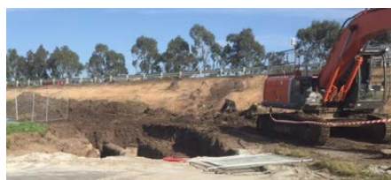
Excavation works to expose a section of a pipeline (top). Preparation works ahead of recoating of a pipeline (centre). Back filling of a section of a pipeline after protection works have been completed (bottom).
