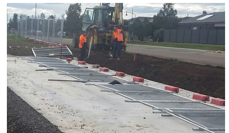
Additional protection works being carried out over a section of a pipeline near a proposed development.
