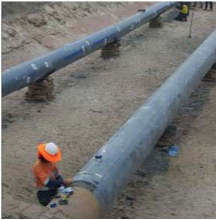
Large scale works may be required as part of additional protection works on pipelines that require substantial forward planning.
