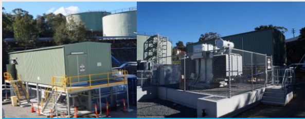
One of the three new substations and transformers.
