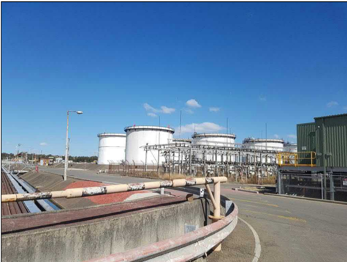
Figure 35: View of MTS1 33kV switch yard looking south west
