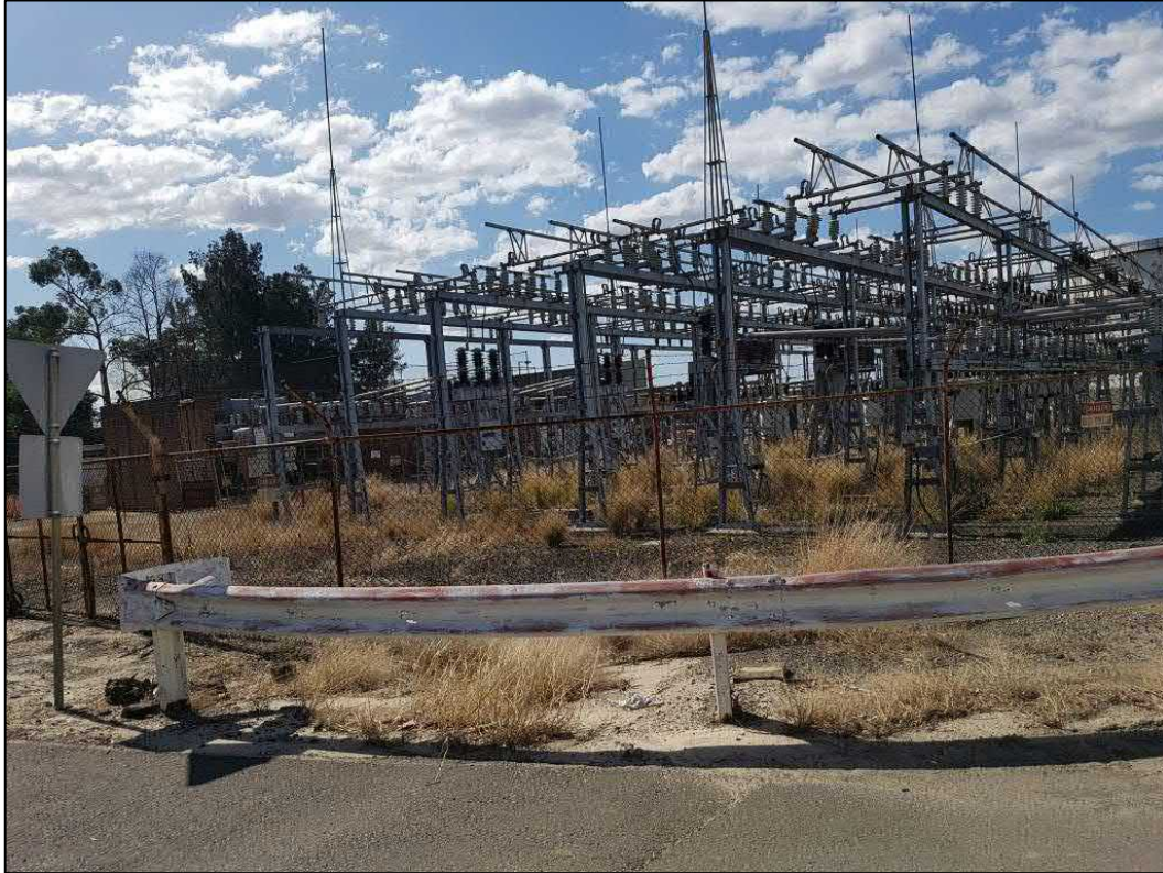
Figure 34: View of MTS1 33kV switch yard looking east
