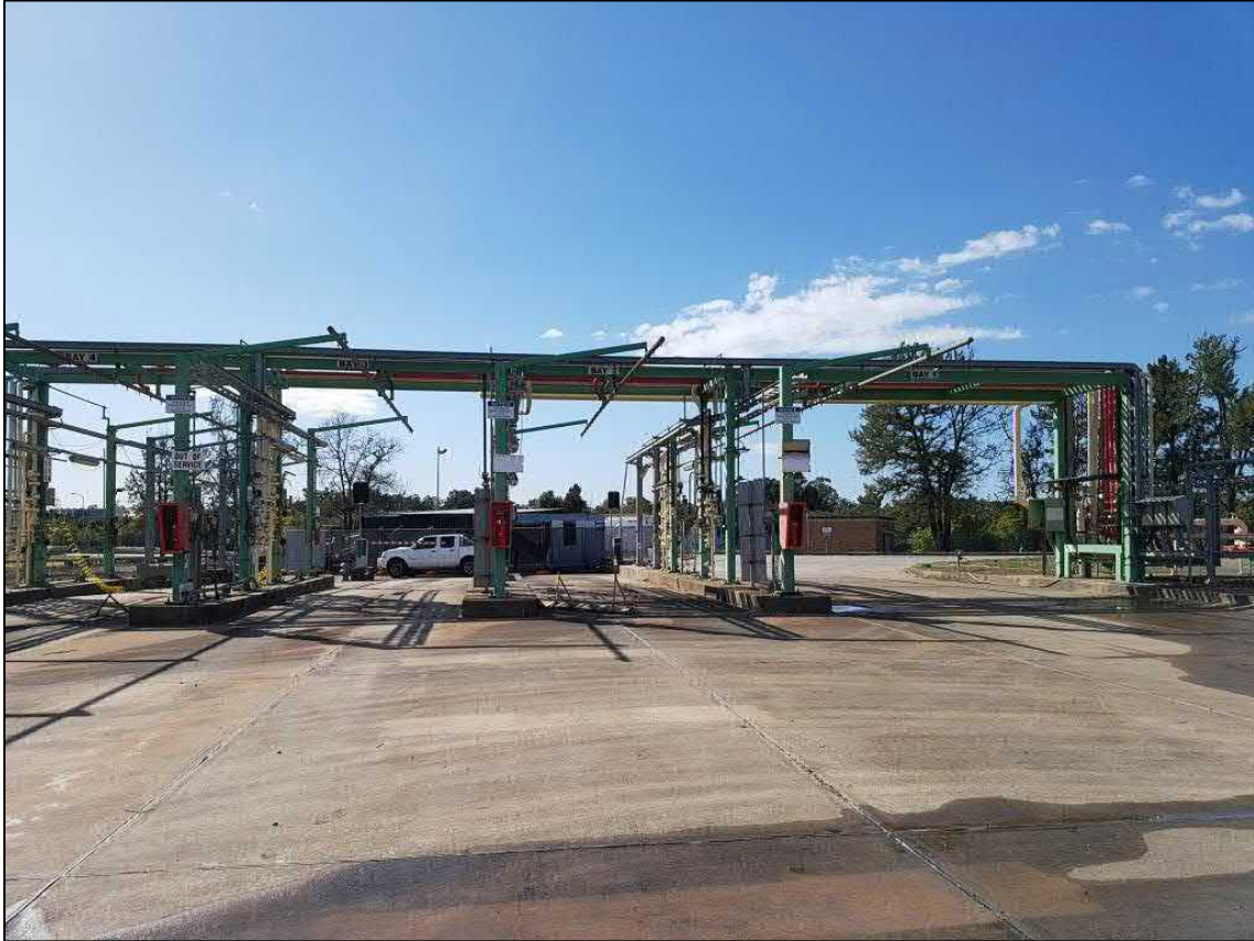
Figure 40: View of LPG truck loading gantry looking north east
